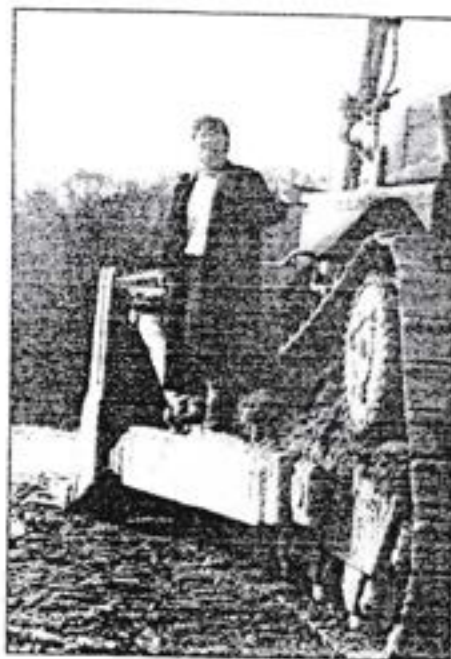
Women's coach Ann Depperman hangs on to the bulldozer being used to construct the new women's soccer field. The field should be completed by Spring of 1993.
